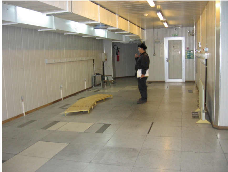
Figure 5: NTT Local Control Room (2nd Floor)
