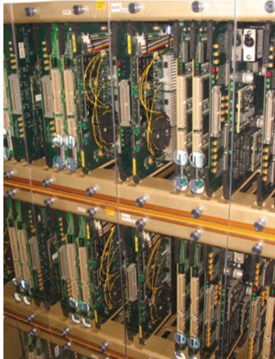
Figure 4. Front panel image of two bins in a Station Electronics rack showing TFB cards, station cards and other system cards (see Correlator Station Electronics in Figure 1). The pairs of holes seen in front of each TFB card allows cool air from the correlator room to be blown into the rack.
