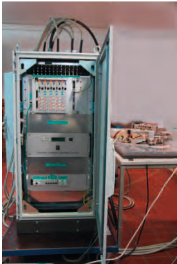
Figure 7. An advanced prototype of one of the final electronics cabinets controlling four of the KMOS pickoff arms during tests at USM.
