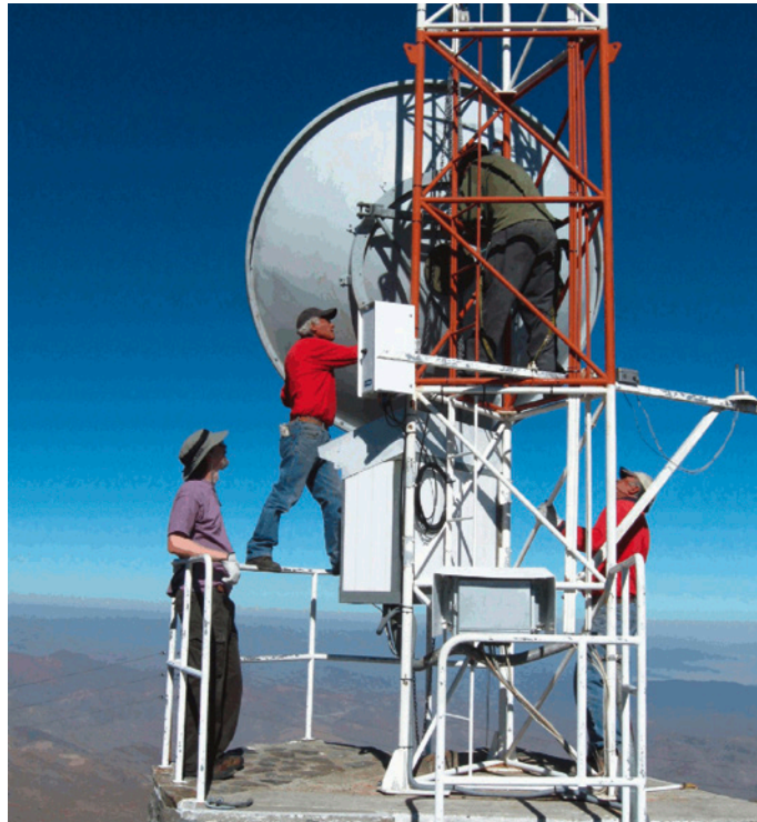
Figure 2. Installation of a 2-metre-diameter radio antenna on the La Silla weather tower. A matching antenna at Cerro Tololo receives the LSQ image data and transmits them to Yale over a high-speed internet link with the USA.
