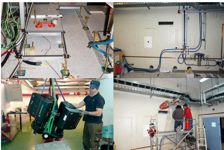
Figure 4. An album of work in progress for the VLTI upgrade: installation of the new false floor covering the cable trays running from the instruments (upper left); installation of a new cooling distribution system in the Combined Coudé Laboratory (upper right); integration of a more powerful pump to provide cooling for the second generation instruments (lower left); drilling of a new feedthrough between the Combined Coudé and the VLTI Laboratories (lower right).
