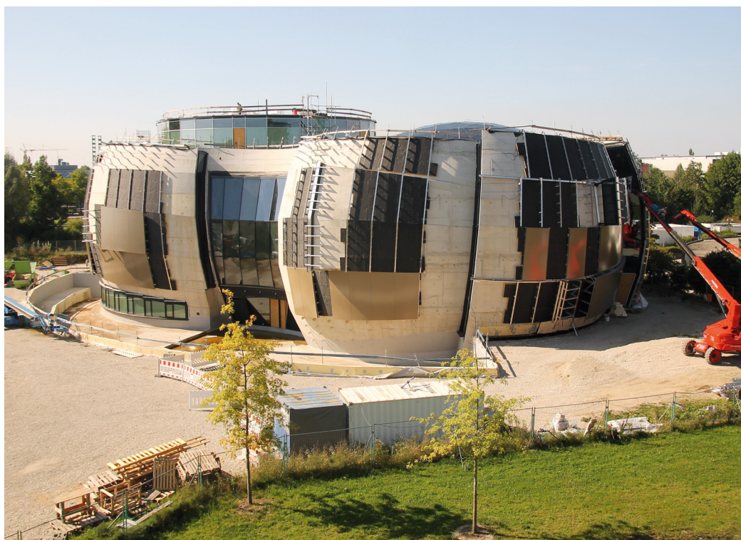
Left: Webcam view of recent construction progress on the ESO Supernova Planetarium & Visitor Centre ( http://supernova.eso.org/ ), due to open in late 2017.
