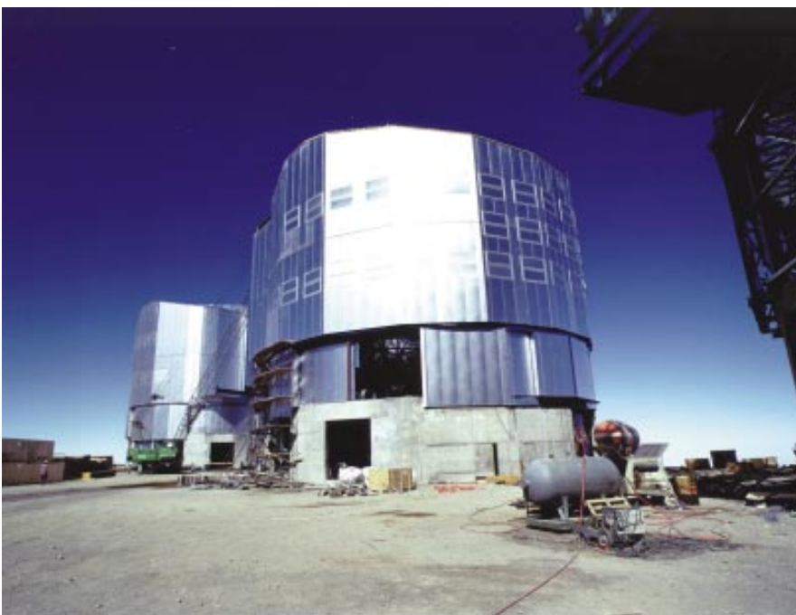
Figure 2 shows details of enclosure no. 2 and in the background enclosure no. 1. Clearly visible are the openings foreseen to optimise the ventilation during the night to avoid any contribution from dome seeing.
