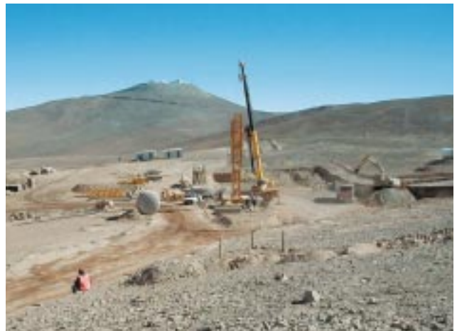
Figure 7: Start of construction. View of the building site where the first part of the new Paranal Residencia and Offices are now under construction.
